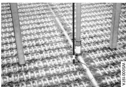
Figure 27: Uniform air discharge
